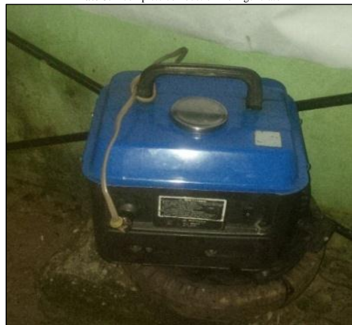
Plate-3. Incomplete combustion from generator
